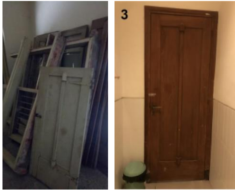
Figure 8. Color comparison of the door leaf before (left) and after (right) conserved. Source: Spasi Architects' (left), 2018 and author's documentation (right), 2022
